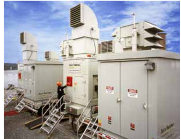
Sited Configuration of Mobile Power Unit
