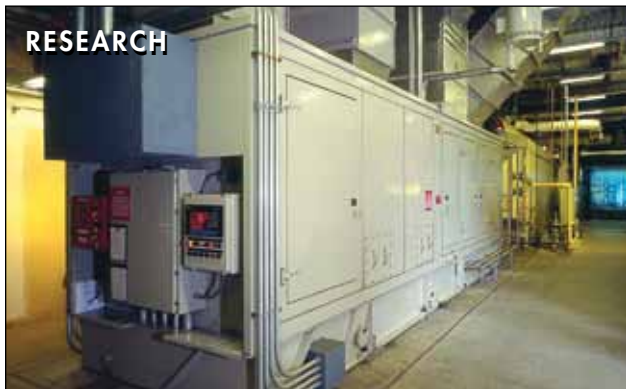
A 5.2 MW Taurus 60 cogeneration system with on-skid controls serves this pharmaceutical research facility in Wallingford, Connecticut, U.S.A.
