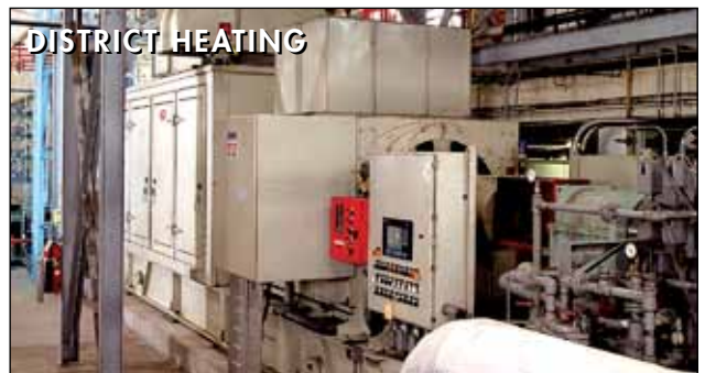
Two 5.2 MW Taurus 60 SoLoNOx generator sets provide district energy to downtown St. Louis, Missouri, U.S.A., as well as electric power to the wholesale market.
