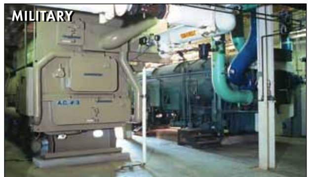
Two 5.2 MW Taurus 60 gas turbines provide cogeneration at this medical center on a United States military base in San Antonio, Texas, U.S.A.
